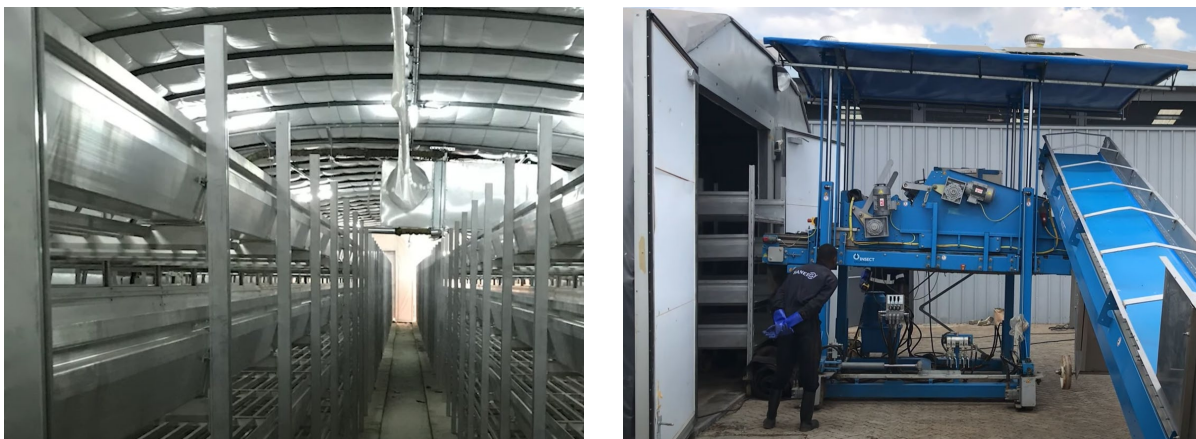
FIGURE 4: LEFT: A BED USED FOR BSF LARVAE REARING. RIGHT: SETTING UP THE MACHINE FOR AUTOMATIC LOADING OF A BED WITH FEEDSTOCK (INSECTENGINEERS).
